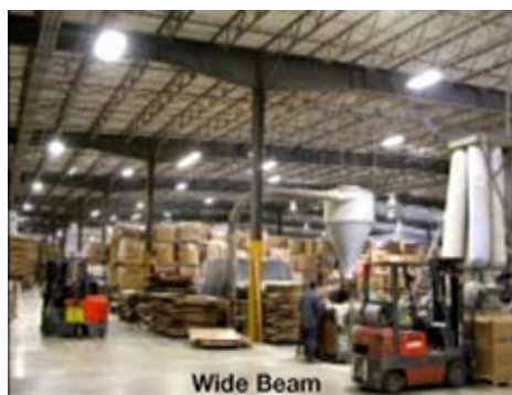
Photo bottom: Wide Beam Fluorescent Lighting
